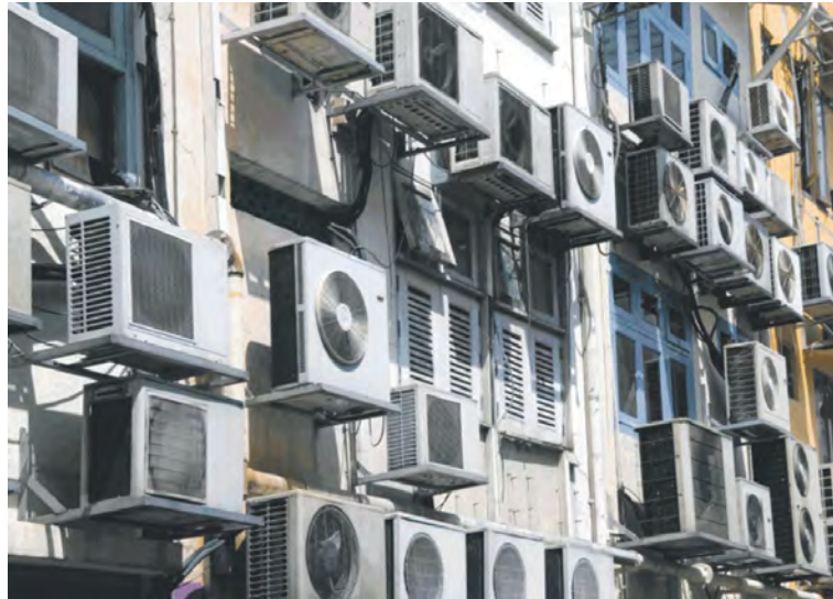
Figure 2.9: An air conditioning unit while using a lot of energy for cooling indoor spaces, actually blows more heat outdoors than it cools indoor
